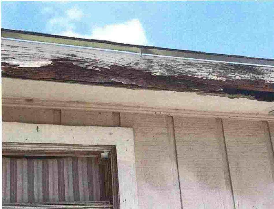
Updated photo taken on June 23, 2026: Roof eaves and soffits are rotten and crumbling.
