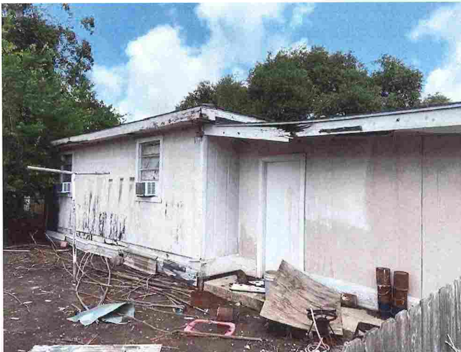
Picture taken 7/29/2020; overhand fascia and trim rotten and partially collapsed, AC window units blocking emergency means of egress, siding rotten and mildewed, rubbish and debris scattered throughout yard providing habitat for pest and vermin
