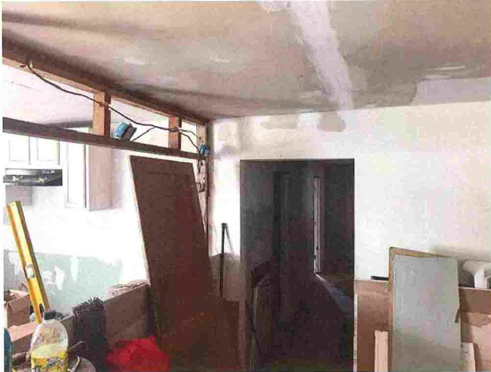
Updated photo taken on June 23, 2026: Walls appear to be in process of being closed in with no open wall inspections, rubbish and debris inside structure causing fire and safety hazards.
