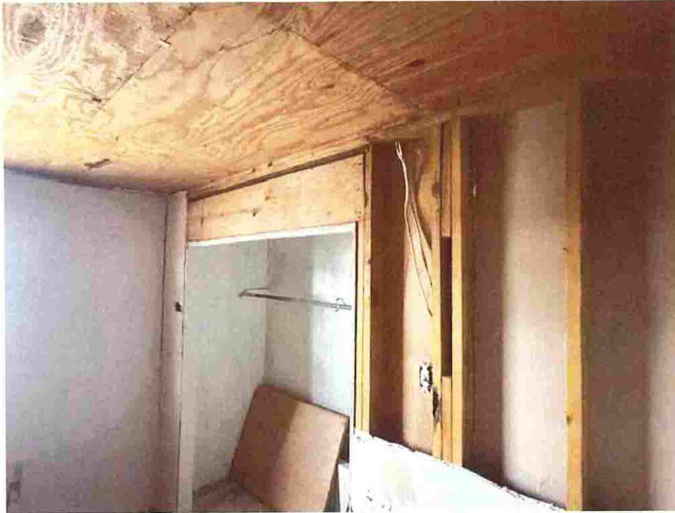
Updated photo taken on June 23, 2026: Exposed electrical wires causing fire and safety hazards. Closing in ceiling and walls with out inspections.
