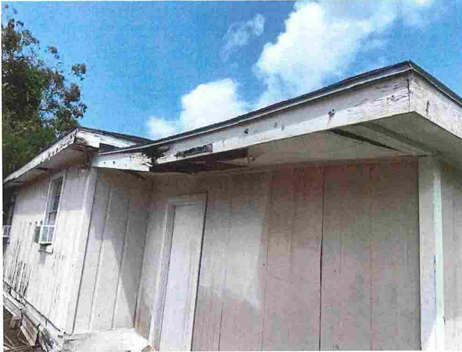
Picture taken 7/29/2020; overhand fascia and trim rotten and partially collapsed, AC window units blocking emergency means of egress.
