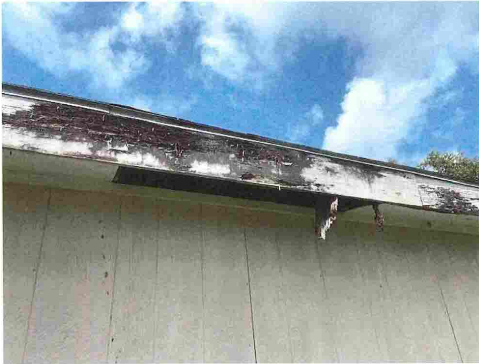
Picture taken 7/29/2020; roof fascia and trim rotten and dilapidated
