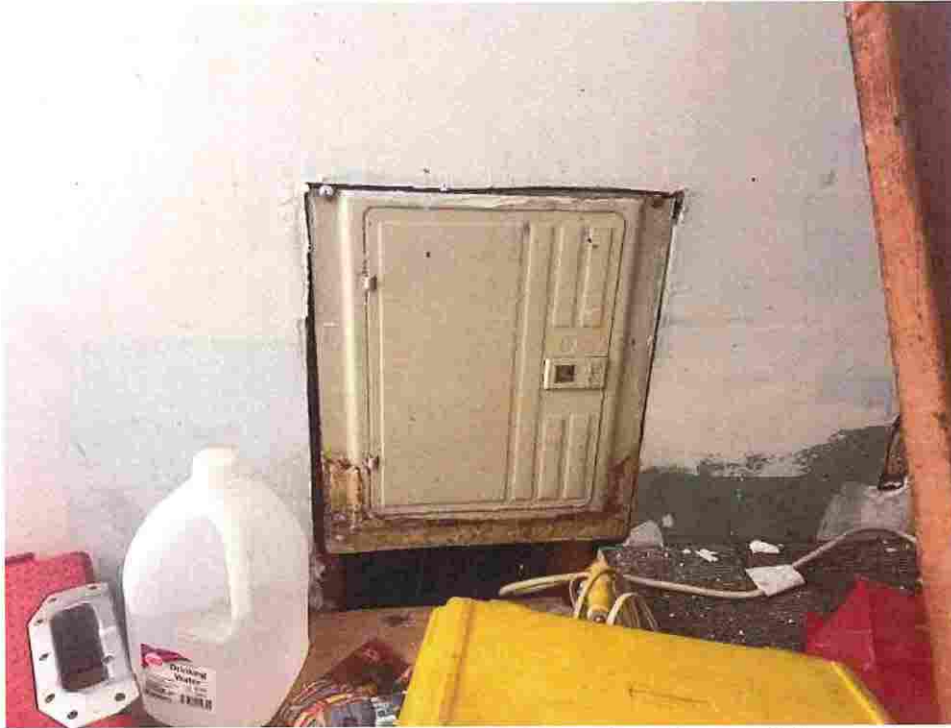
Updated photo taken on June 23, 2026: Interior of state of disrepair, exposed electrical wires causing fire and safety hazards.
