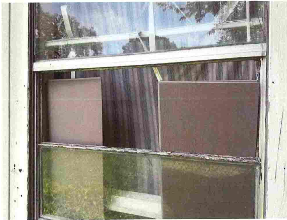
Updated photo taken on June 23, 2026: Window is ajar allowing moisture and the elements to freely enter structure leading to further deterioration.
