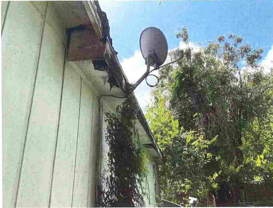
Picture taken 7/29/2020; roof fascia and trim rotten and dilapidated, vines overgrowing structure causing structural damage
