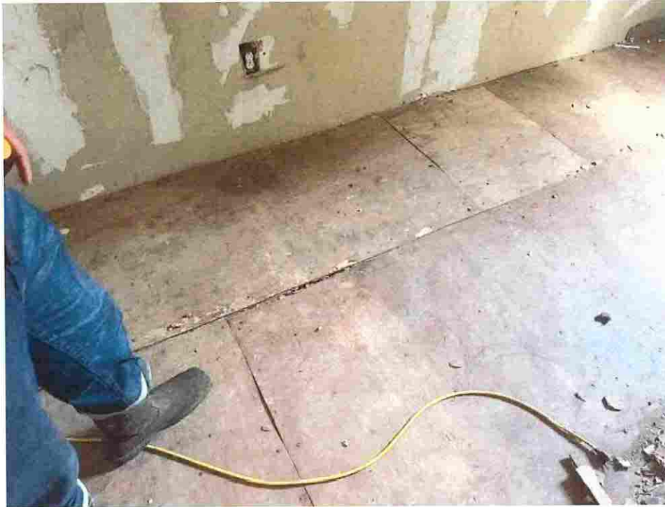
Updated photo taken on June 23, 2026: Missing floor, sub floor rotten in some areas, extension cord causing fire and safety hazards.
