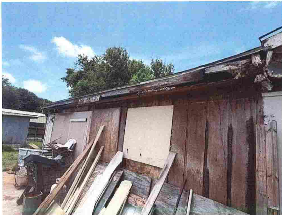
Updated photo taken on June 23, 2026: Loose construction material at risk of blowing away in high wind event causing damage to neighboring properties, roof soffits and eaves damaged and rotten, side of building missing siding with large gaps allowing moisture and the elements to freely enter structure.
