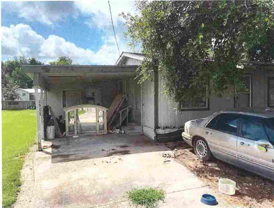
Picture taken 7/29/2020; siding and trim rotten and dilapidated, rubbish and debris piled under carport proving habitat for pest and vermin, junked car abandoned on property
