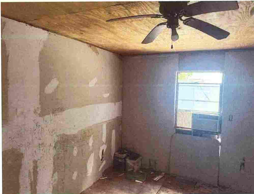
Updated photo taken on June 23, 2026: Missing floor, sub floor rotten in some areas, hole in wall can see day light.
