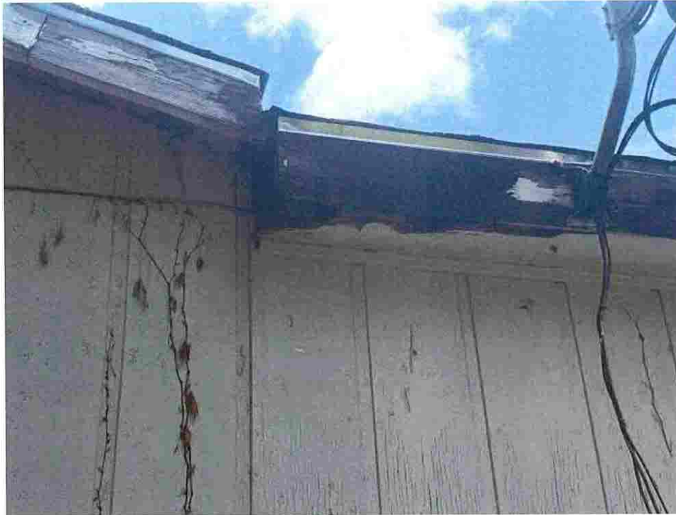
Updated photo taken on June 23, 2026: Roof eaves and soffits rotten foliage growing into structure.
