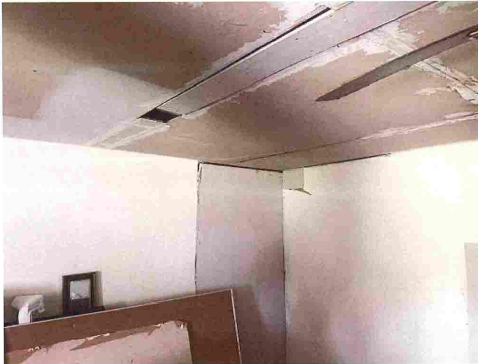
Updated photo taken on June 23, 2026: Walls appear to be in process of being closed in with no open wall inspections, rubbish and debris inside structure causing fire and safety hazards.
