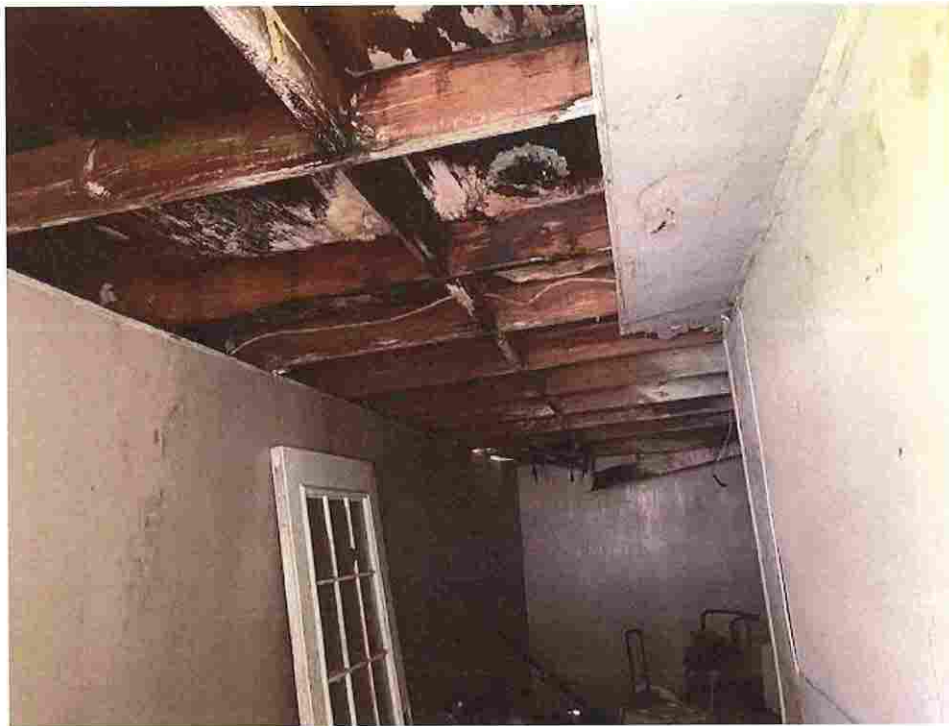
Picture taken 7/29/2020; insulation and ceiling covering missing, severe water damage and mold present on ceiling causing rot, exposed electrical wiring run through ceiling
