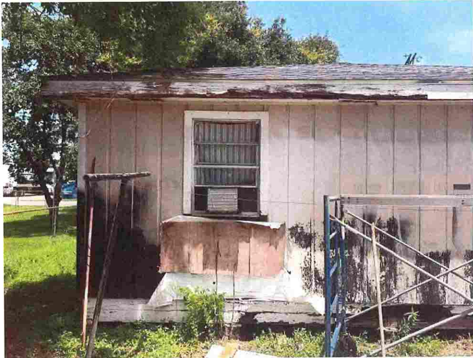
Updated photo taken on June 23, 2026: Roof eaves are severely rotten and mildewed, exterior siding stained, peeling away and damaged, foundation sills also showing signs of rot, window unit not weatherproof allowing moisture to enter structure.
