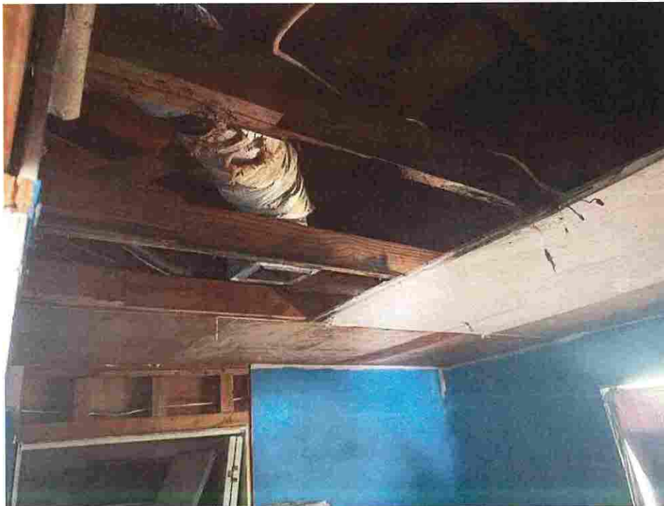
Updated photo taken on June 23, 2026: Exposed electrical wires causing fire and safety hazards. Ceiling joist appear to be rotten will not meet span table.
