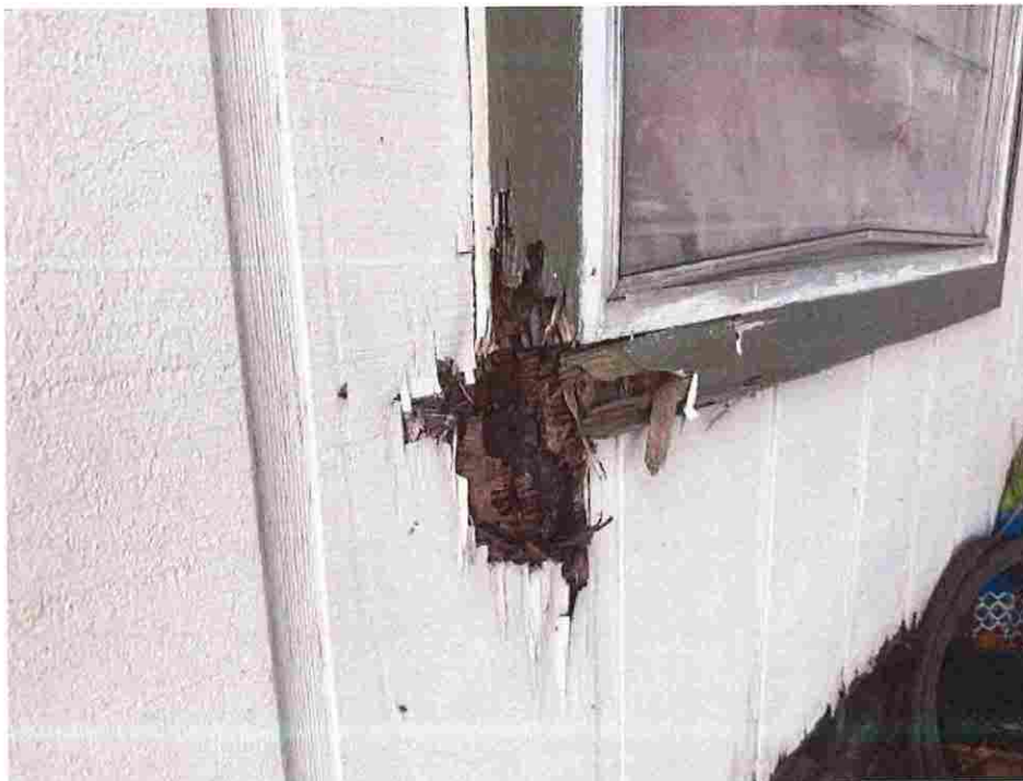
Updated photo taken on June 23, 2026: Exterior siding and window sills are severely rotten and crumbling.
