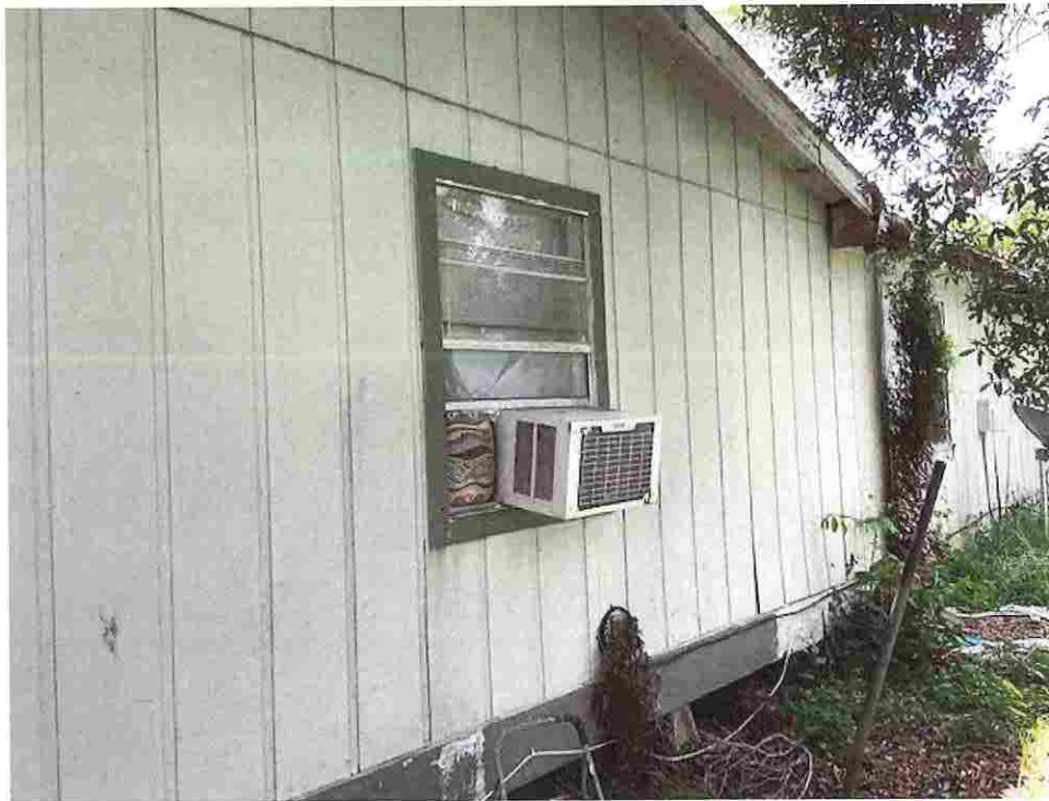
Picture taken 7/29/2020; window unit blocking emergency means of egress, siding, fascia and trim rotten and dilapidated, exposed electrical wiring running along exterior of structure
