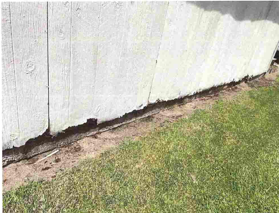
Picture taken 7/29/2020; siding rotten and crumbling
