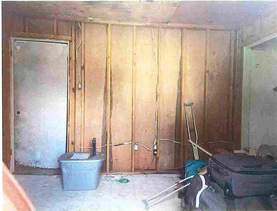
Picture taken 7/29/2020; insulation and wall covering missing from interior of home, exposed electrical wiring run all throughout interior
