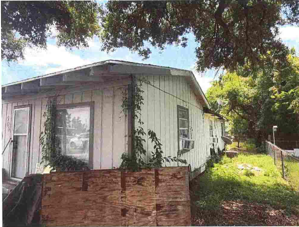
Updated photo taken on June 23, 2026: Foliage growing into structure, loose construction material at risk of blowing away in high wind event causing damage to neighboring properties, roof soffits and eaves damaged and rotten.
