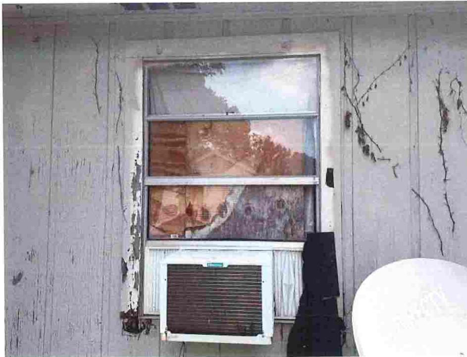
Updated photo taken on June 23, 2026: Window unit not weatherproof allowing moisture to enter structure.
