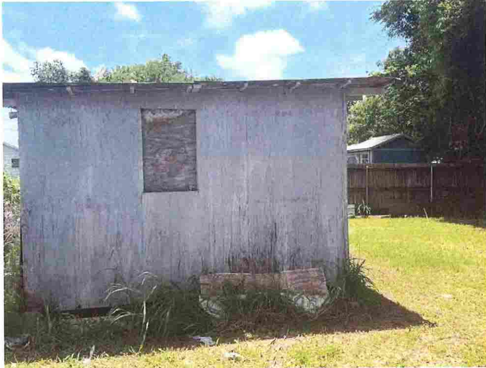
Updated photo taken on June 23, 2026: Overgrown foliage, accessory structure not maintained.
