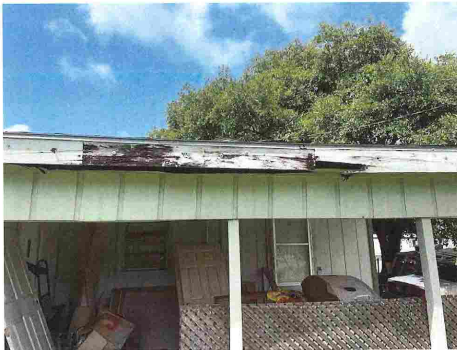
Picture taken 7/29/2020; roof fascia and trim rotten and dilapidated, rubbish and debris scattered throughout property and piled under carport, providing habitat for pest and vermin.
