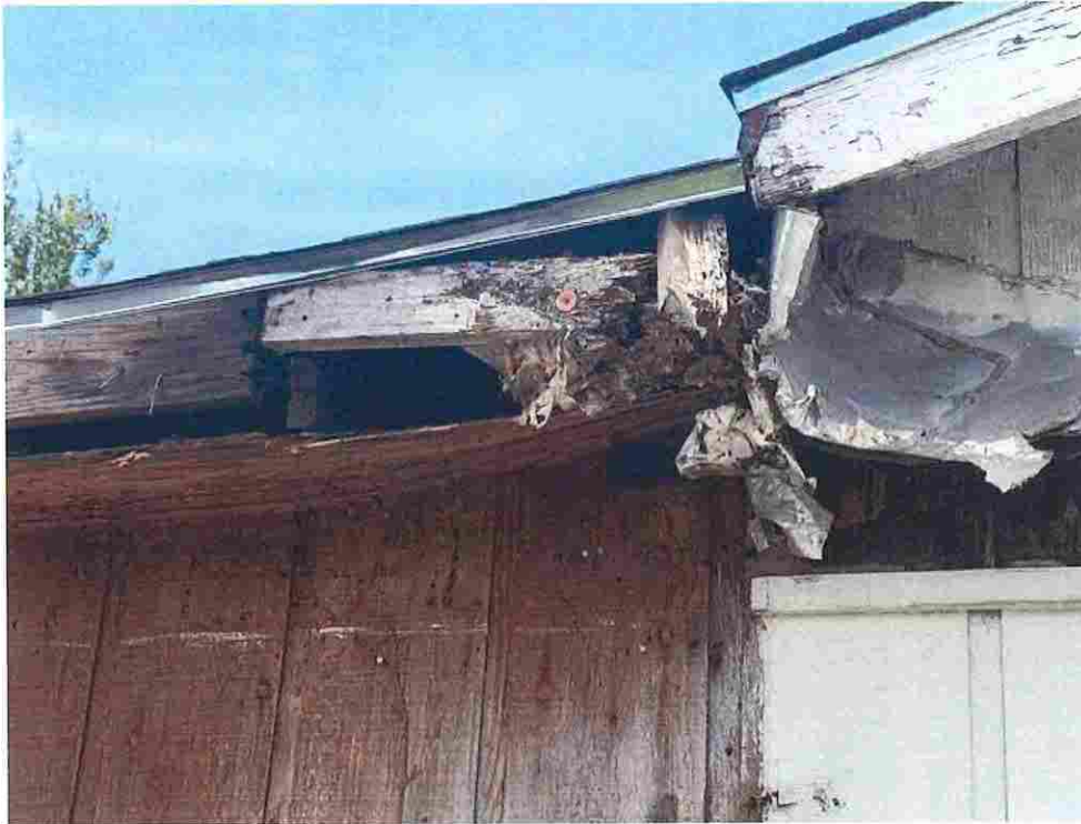
Updated photo taken on June 23, 2026: Roof eaves and soffits severely rotten and crumbling with large gaps open to the elements causing further deterioration.
