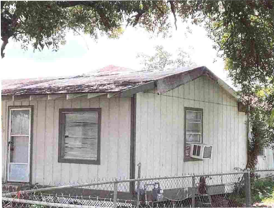
Picture taken 7/29/2020; roof structure damaged and rotten exposing interior to water damage, AC window unit blocking emergency means of egress
