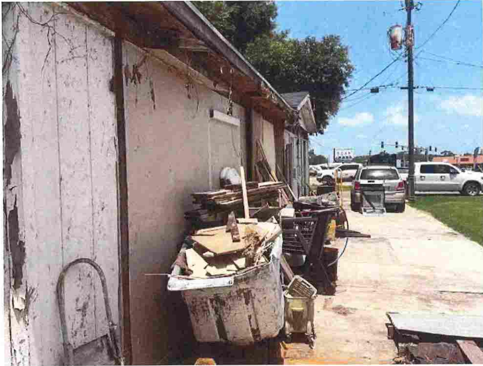
Updated photo taken on June 23, 2026: Missing exterior siding causing blighting, construction debris and material causing blighting and at risk of blowing on neighboring property in high wind event causing damage, vines growing into structure, roof eaves and soffits rotten and damaged.
