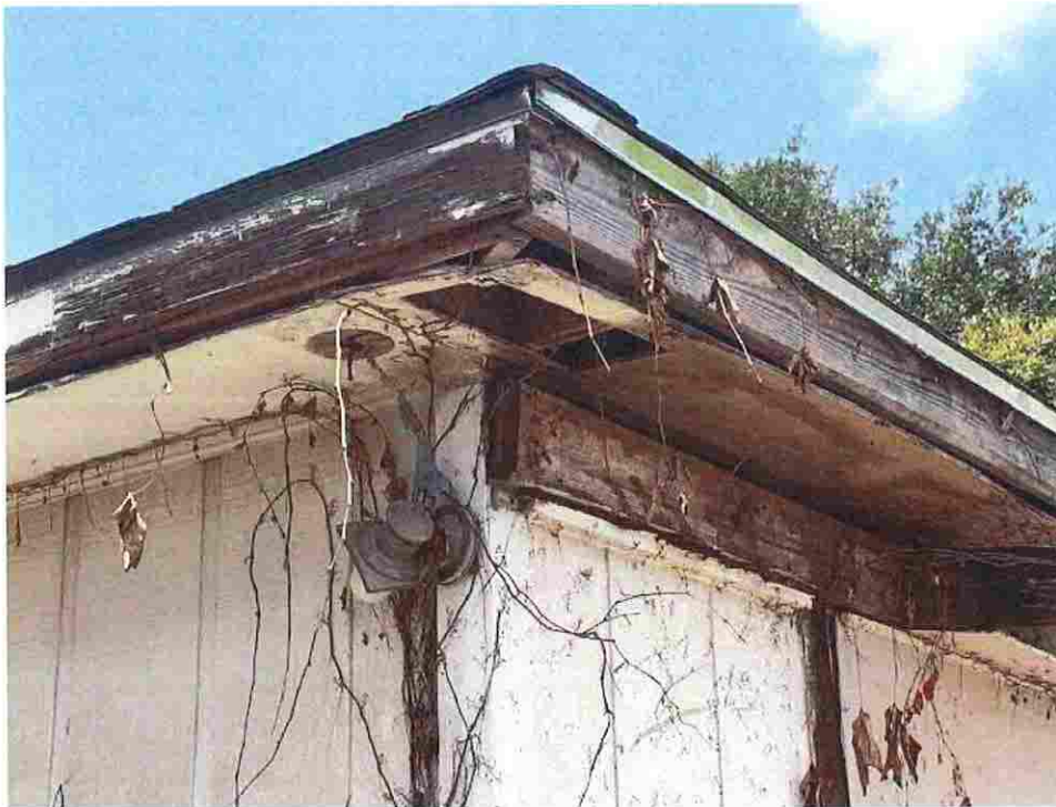
Updated photo taken on June 23, 2026: Exposed electrical wiring from hanging and damaged light fixtures causing fire and safety hazards, vines and foliage growing into structure, roof eaves and soffits are rotten and damaged with large gaps allowing moisture to enter leading to further rot.
