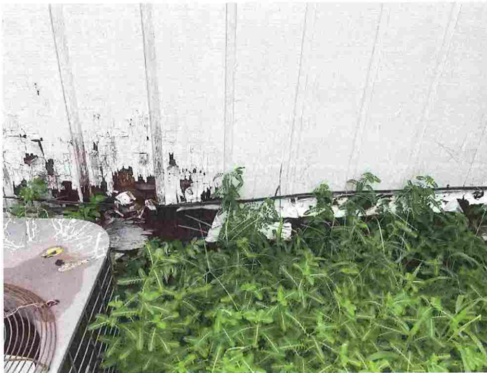
Picture taken 7/29/2020; siding rotten and crumbling from moisture damage, grass and weeds overgrown providing habitat for pest and vermin
