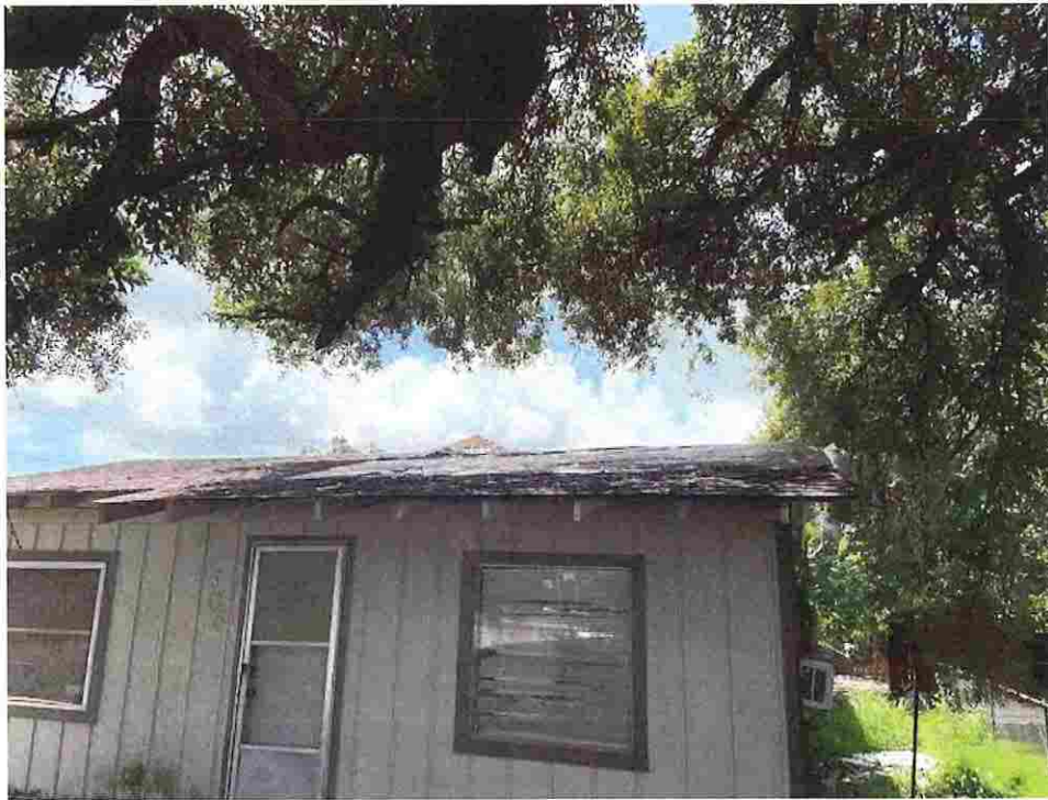
Picture taken 7/29/2020; roof structure damaged and rotten exposing interior to water damage, AC window unit blocking emergency means of egress, grass and weeds overgrown providing habitat for pest and vermin
