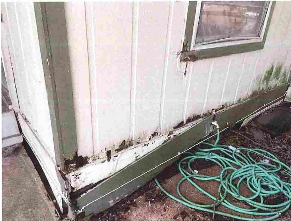
Picture taken 7/29/2020; siding and trim rotten and dilapidated from moisture damage
